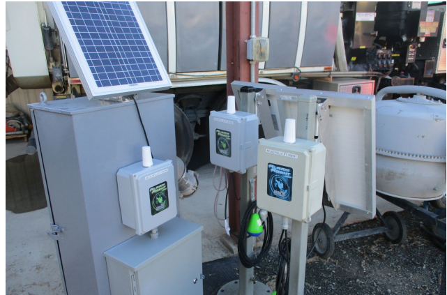
Lake County has mounted their units so they are portable.
